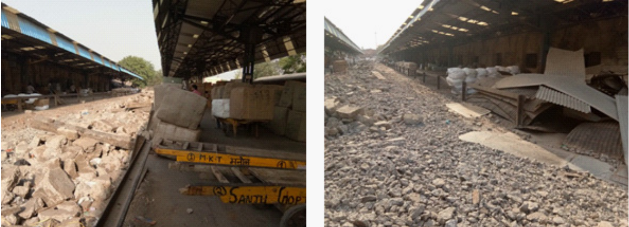
Figure 33: Photographs showing the poor condition of access points for parcel holding/loading areas at the Old Delhi Station (May 1, 2018)
