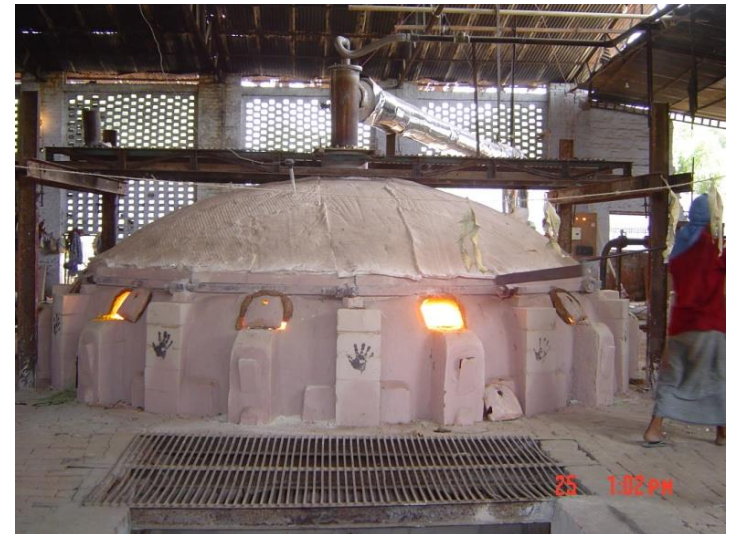
Recuperative Natural Gas fired Pot Furnace
