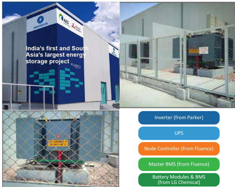
FIGURE 12: Grid-connected BESS in Rohini, Delhi
