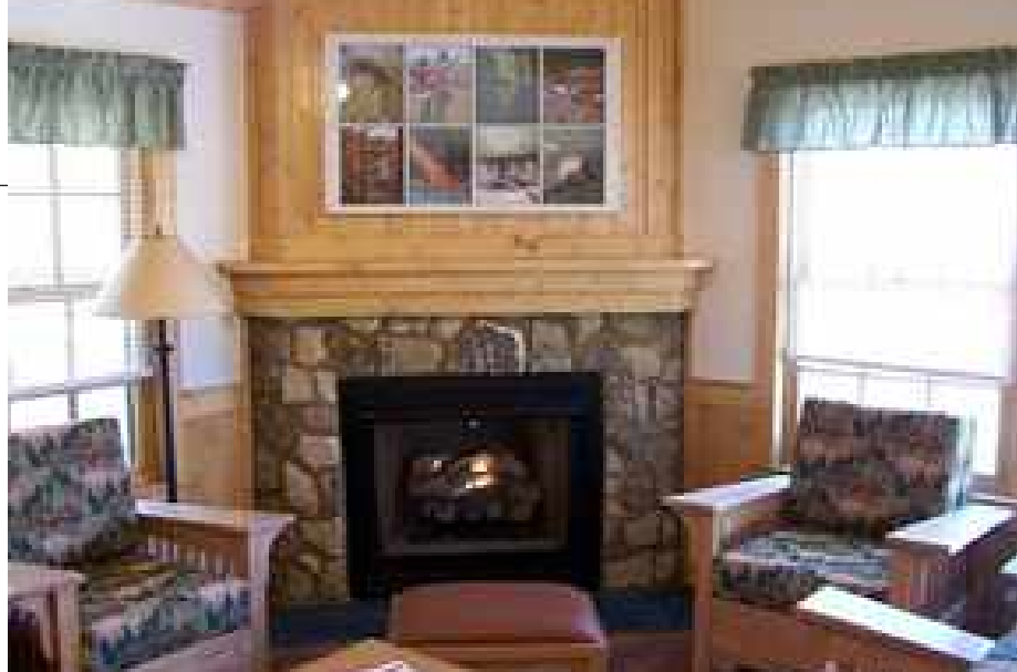
A gas-powered fireplace and fireplace vents
