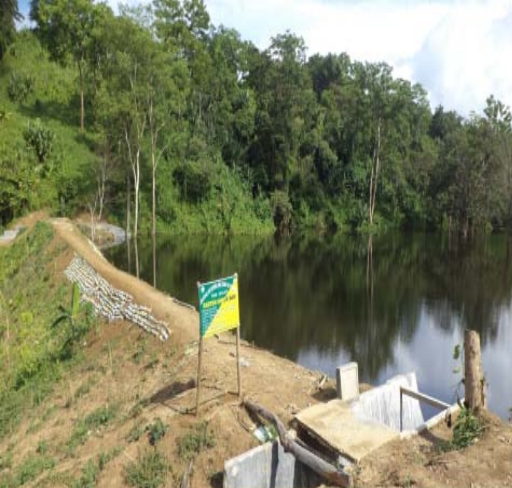
Name of Project: North Tripura IWMP-II (2010-11) Location: Barahaldicherra /Dasda/Kanchanpur District : North Tripura GPS Coordinates: 24.14266 ° N, 92.22272 ° E Type of Activity: Water Harvesting Structure
