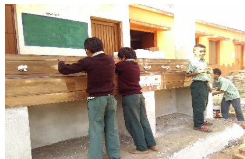
Students at the drinking water station constructed as part of Project FLOW
