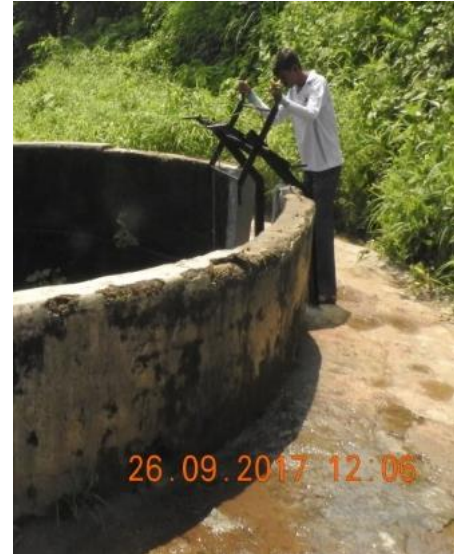
Picture No. 12: A newly installed pulley on one of the wells
