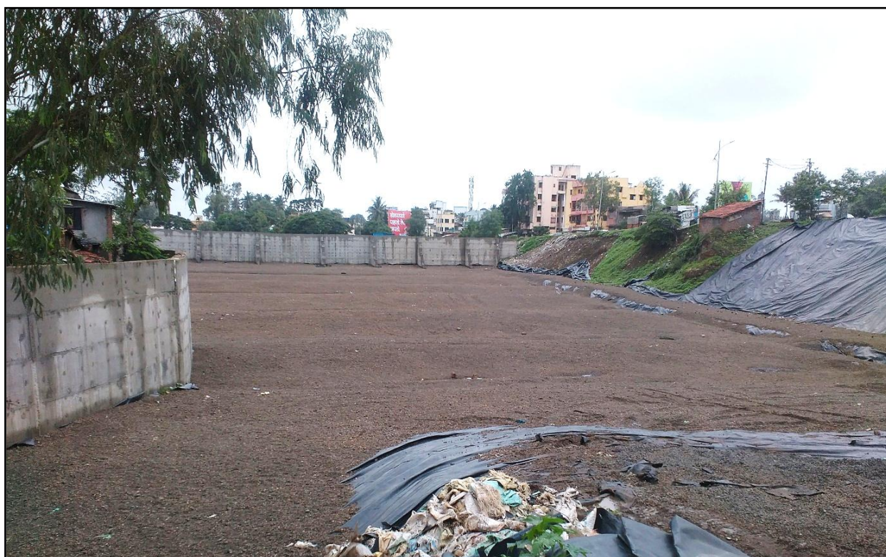
Picture No. 19: The Takala Land fill site layered with HDPE and concrete wall along the periphery Photo credits: TERI
