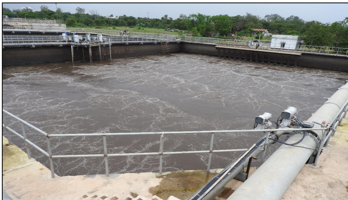
Picture No. 11: One of the basin at the 76 MLD capacity Sewage Treatment Plant at Kasba Bawda Photo credits: TERI
