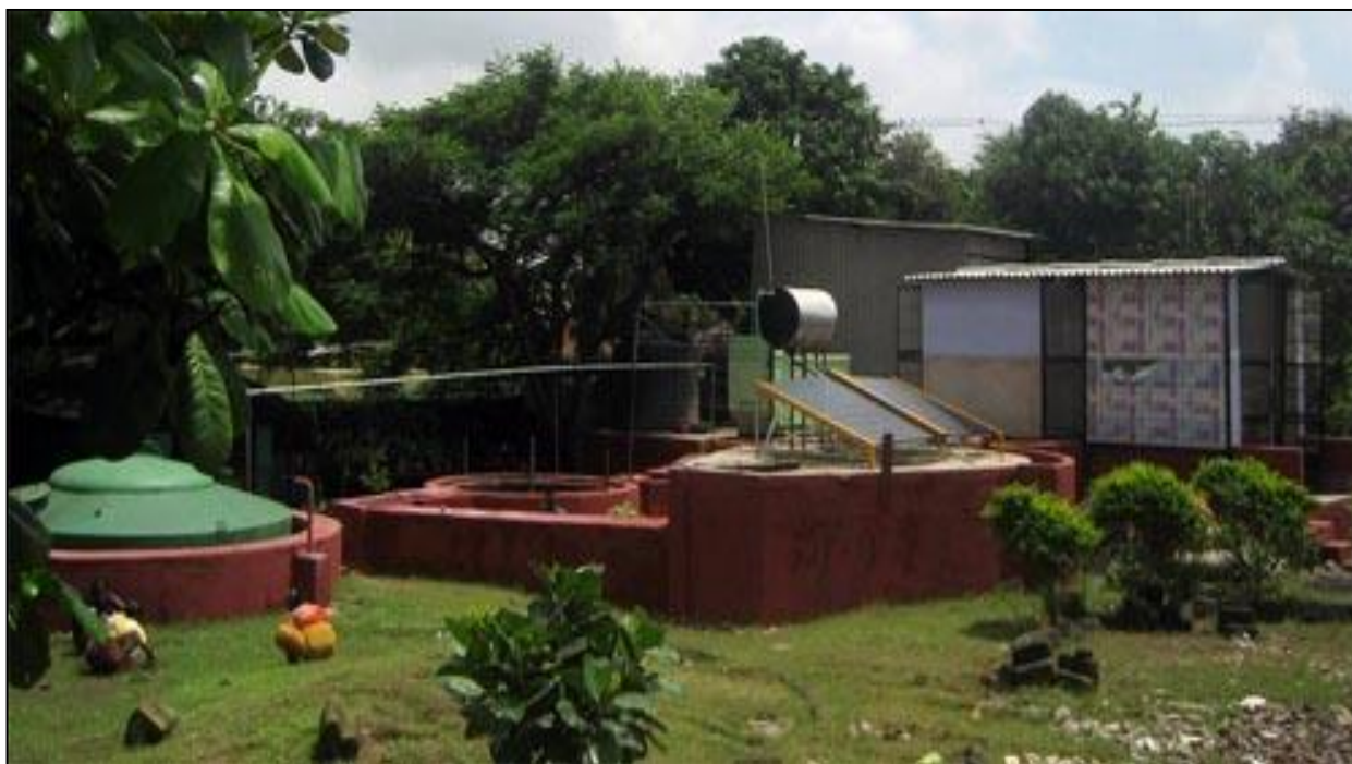
Picture No. 20: Picture depicting a prototype of Bio –Methanation plant Photo credit: KMC
