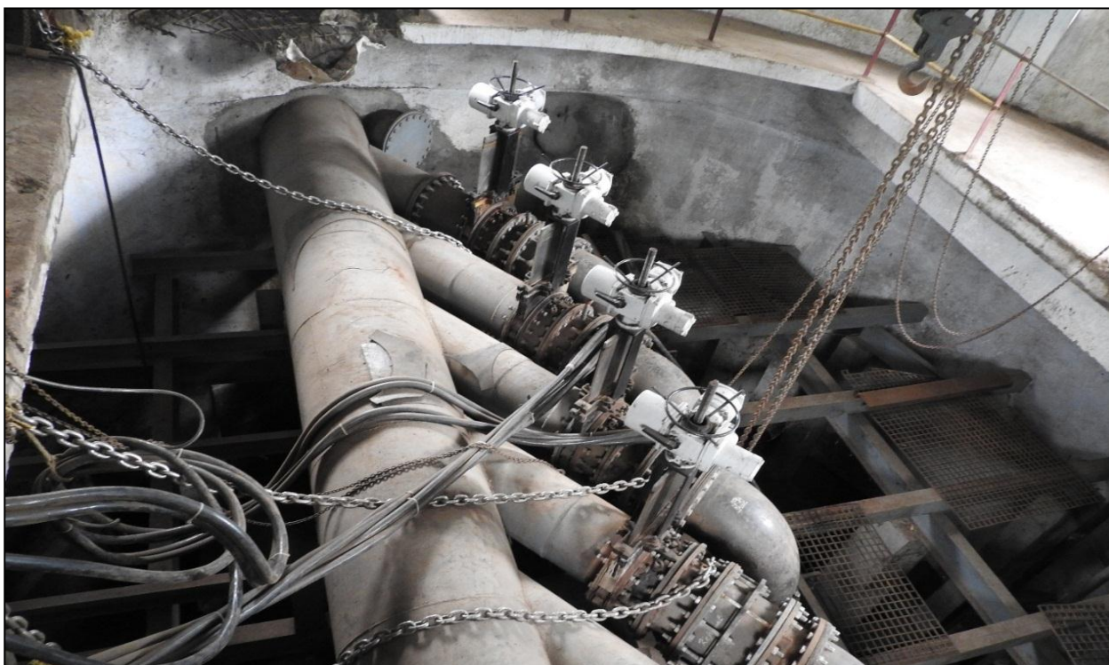
Picture No. 13: Jayanti Nallah pumping station Photo Credit: TERI
