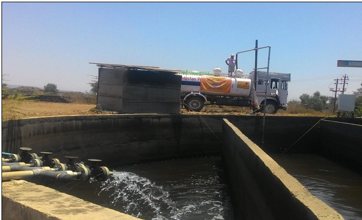
Picture No. 15: Tanker being refilled with treated water for secondary applications at Bawda STP Photo credit: KMC
