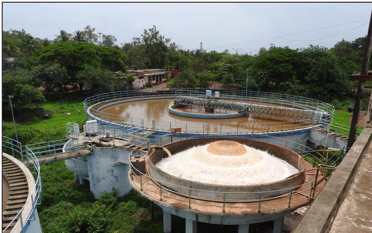
Picture No. 10: The 36 MLD Water Treatment Plant at Kasba Bawda Photo Credit: TERI
