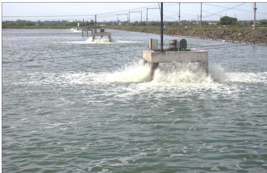
Picture No. 6: The aerated Lagoon at Bondar STP – Nanded City
