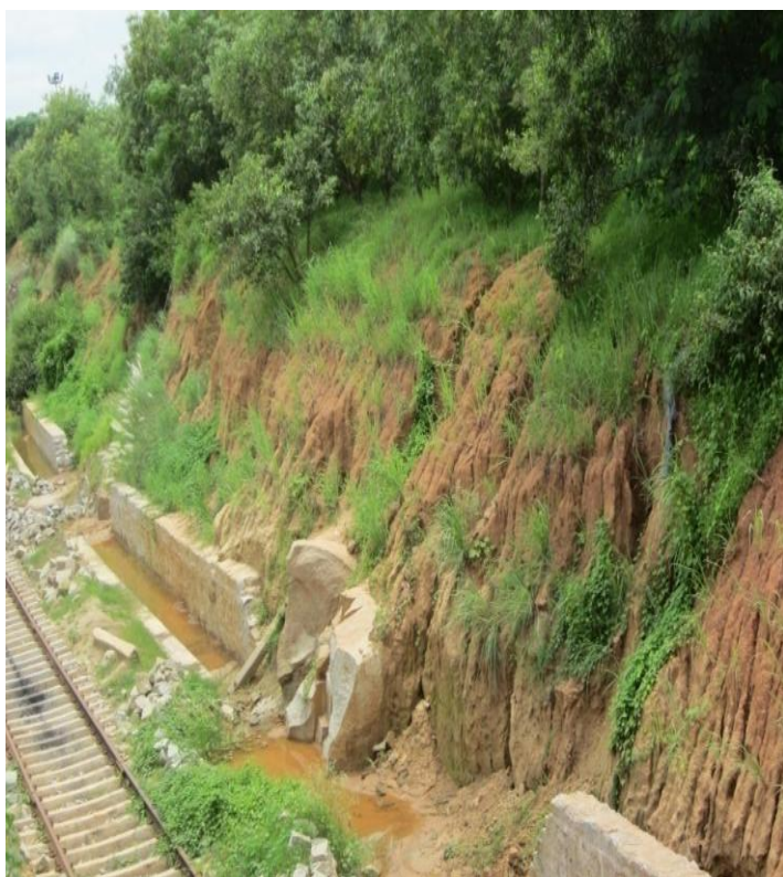
Figure 25 Construction of toe wall & planting of Cymbopogon tufts at railway siding track slope
